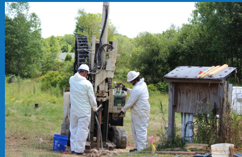
Cascade Technical Services crews provide calculated injections to remediate soil and groundwater contamination
